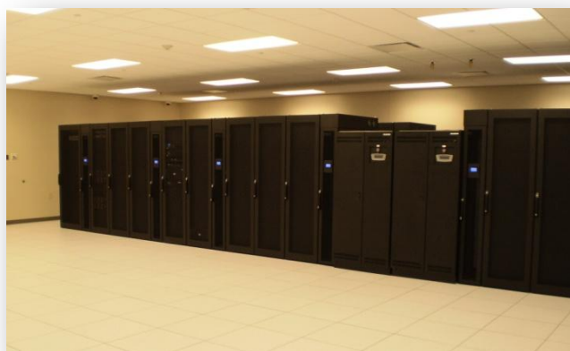
The new Licking Memorial Hospital Data center
